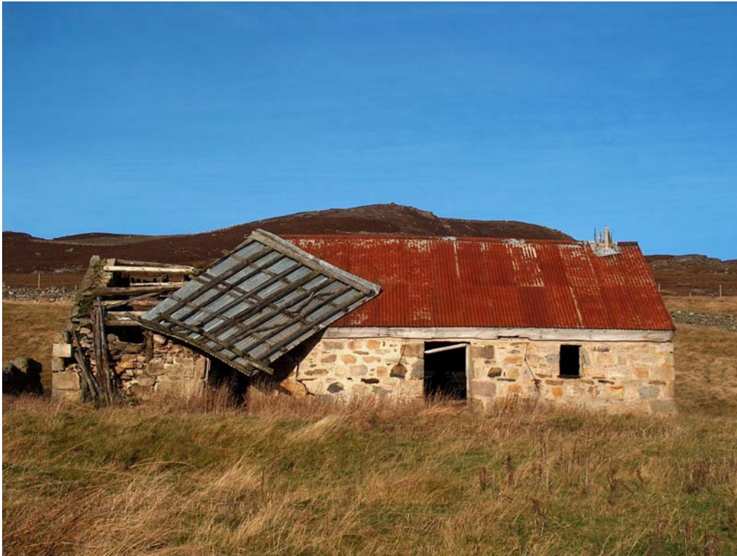
Fig 2 Auchtavan Cottage showing weather damage to left end.
